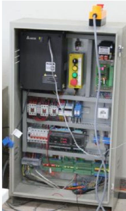
Figure 1 Control cabinet of PLC and inverter
